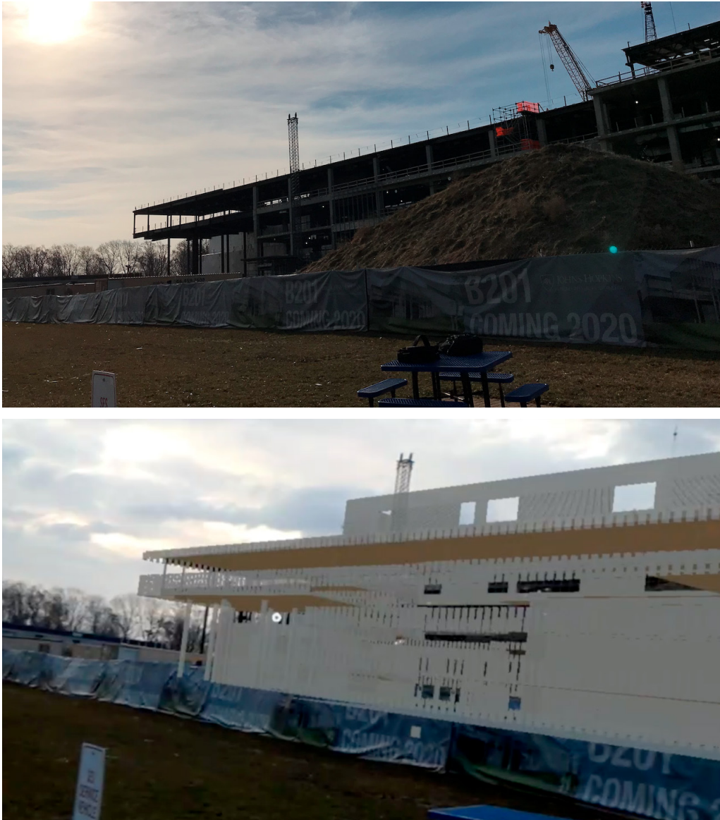
Figure 3. Successful model of B201 in the context of its location. The top image shows the construction site, and the bottom image shows the 3-D model positioned to the construction site.
