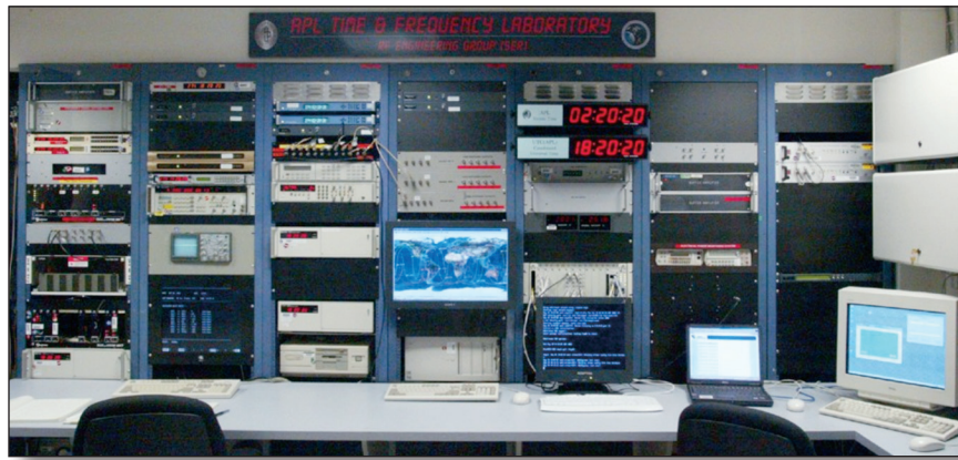
Figure 2. APL’s TFL (building 4, third floor) is a member of the international ensemble responsible for UTC.
