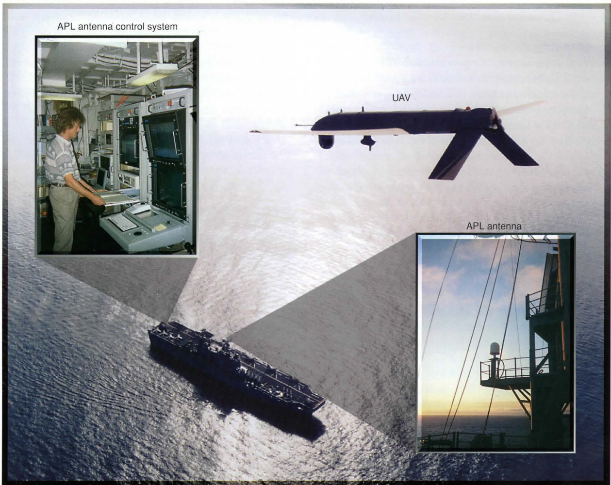
Figure B2-5. APL UAV Tactical Control System antenna installation onboard USS Tarawa .
