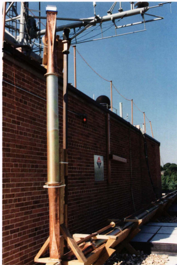
Figure 22. Sixty-foot C-band waveguide run located on the roof of APL's Building 11.
