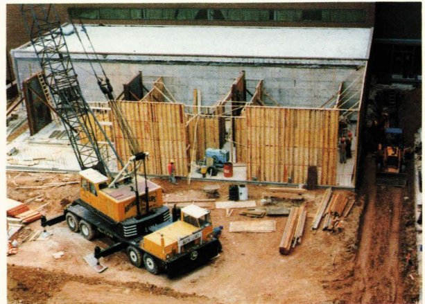
Figure 18 — The Johns Hopkins radiation therapy wing under construction. The high-energy and high-flux levels of the therapy machine demand extraordinary shielding measures. To protect technologists and the general public, the Varian CLINAC-20, which produces 15-MeV X rays at rates up to 300 rads/minute, requires 8 inches of steel embedded in 66 inches of concrete. The radiation barriers in the Johns Hopkins Oncology Center reduce ambient radiation levels to a factor of 10 less than national regulations. Technologist exposure is comparable to that produced by natural background.
