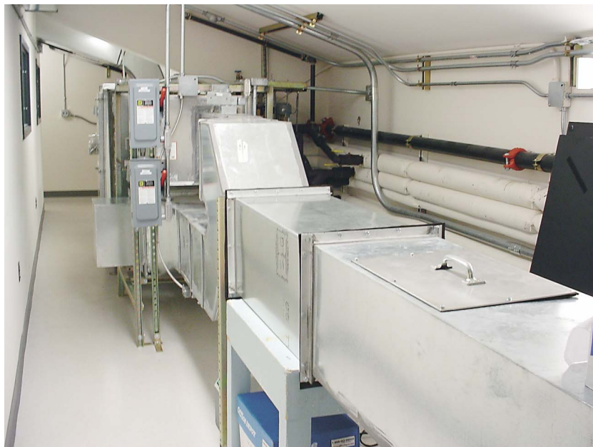
Figure 2. The supply side of the HVAC system for the aerosol test bed in the CBTEC.
