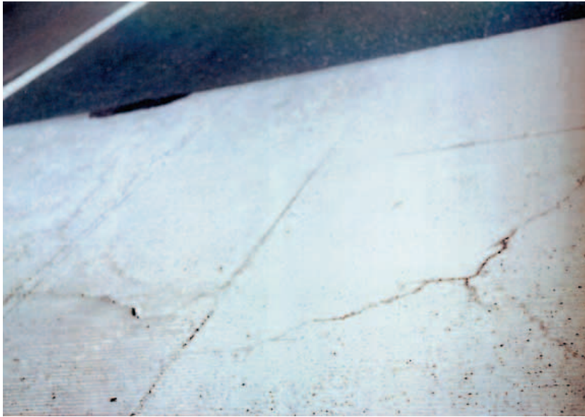
Figure 7. Cracks found on the bridge in Fig. 4. Regions of low CP current in Fig. 6 can be matched with locations of cracks on the bridge deck.
